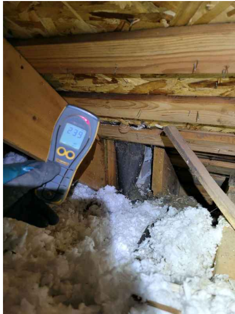
Elevated moisture reading
