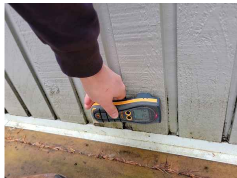
Elevated moisture reading
