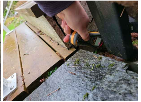
Elevated moisture reading
