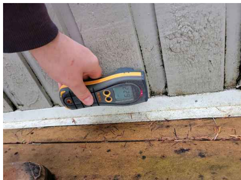
Elevated moisture reading
